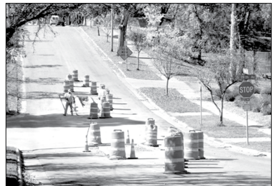
Medians being constructed at 19th Ave. S. to help pedestrians cross 40th St. to get to Sibley Park. The stop sign will be removed.
